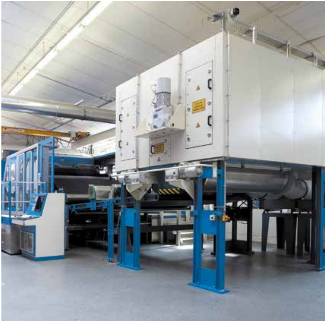
High-performance thermobonding line
